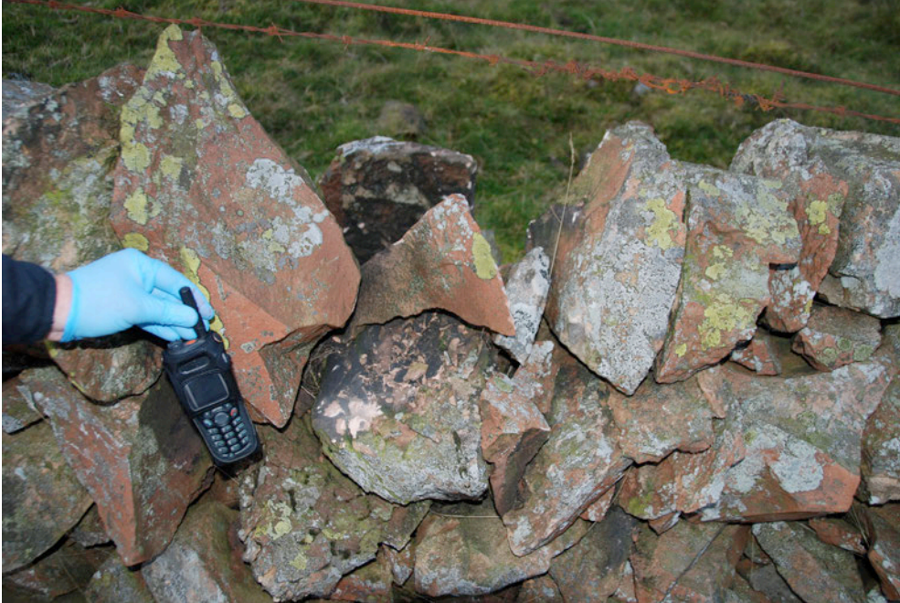
Photo 1, showing damage to wall with police radio shown for scale.
